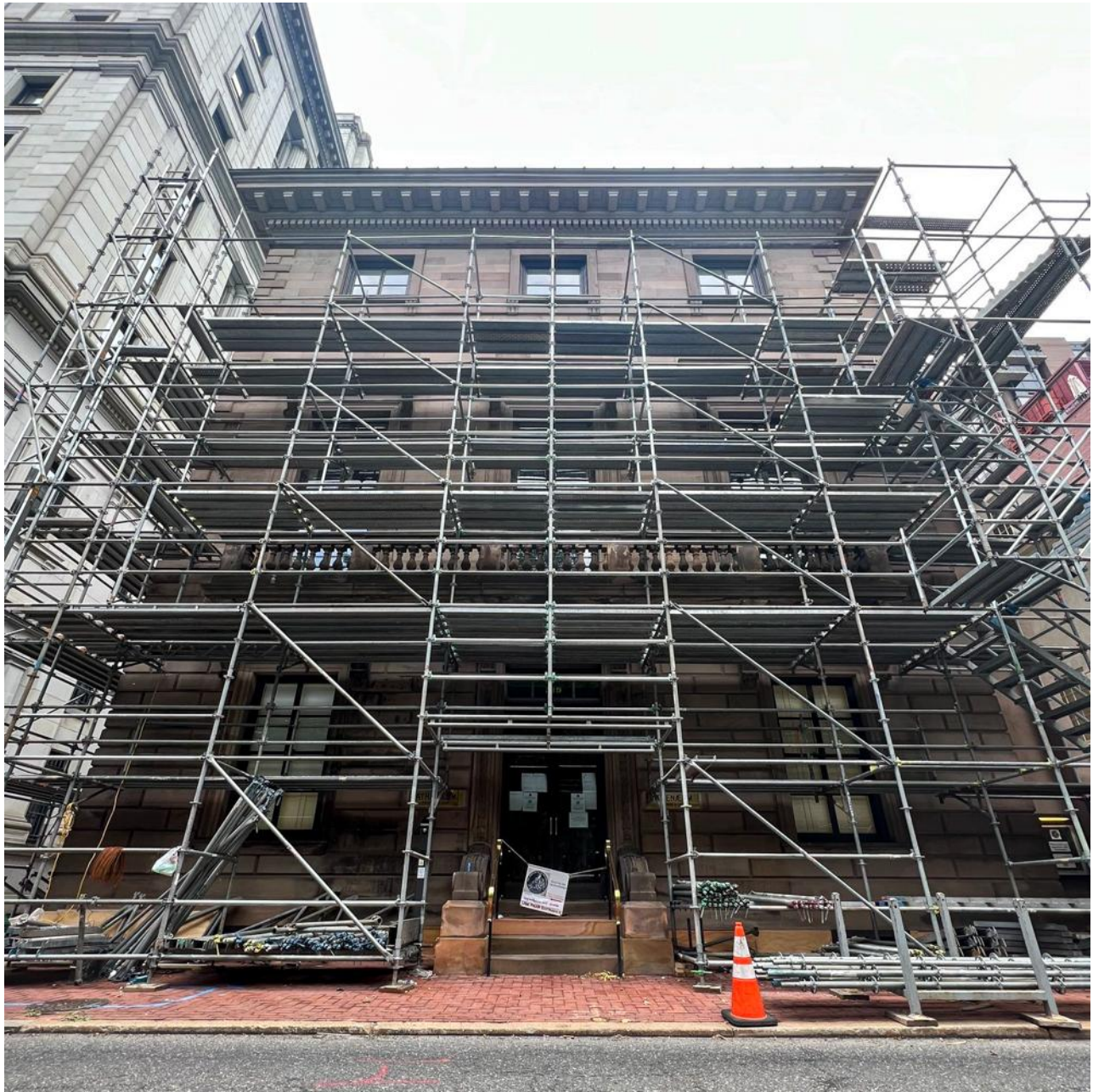
The Athenaeum during facade renovation in 2022. | Photo courtesy of Premier Building Restoration, Inc.
